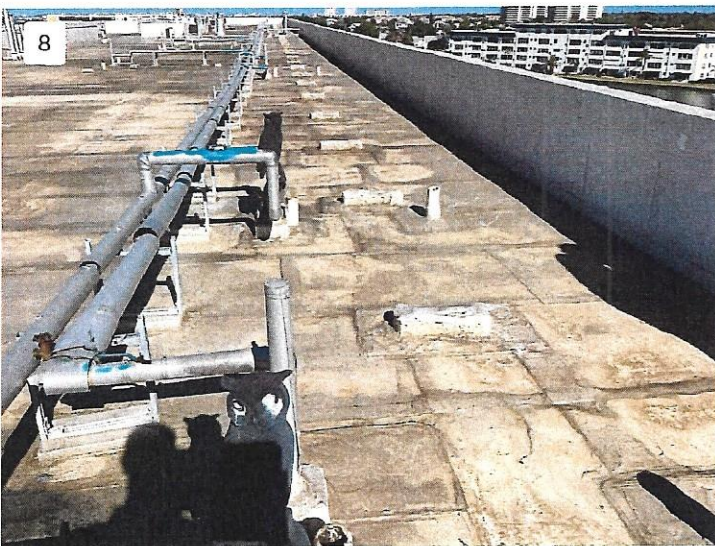
Piping and abandoned stands
