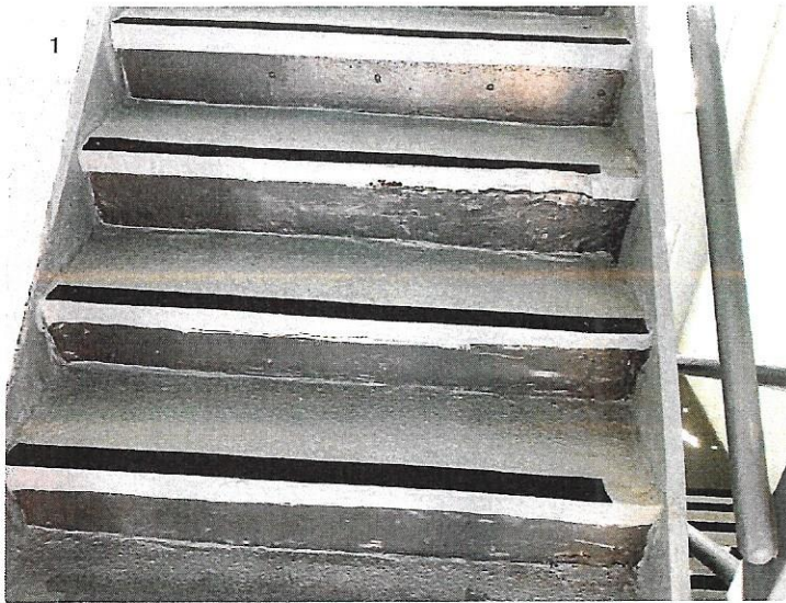
Corrosion of stairs
