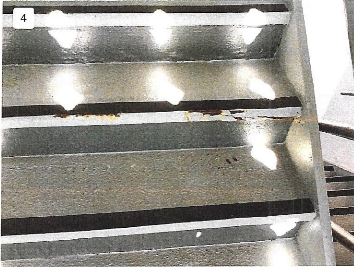
Corrosion of stair tread
