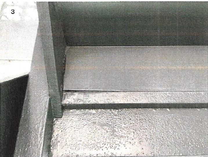
Previous repair of stair tread
