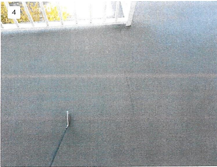
Crack in floor coating at joint
