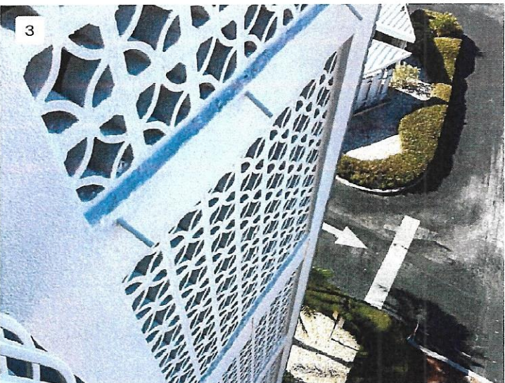
Landing drains in stairwell
