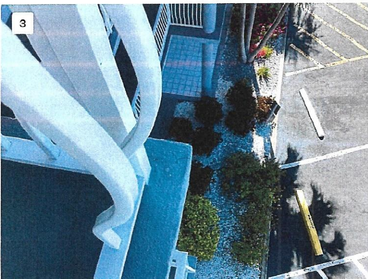
Crack in area of post pocket
