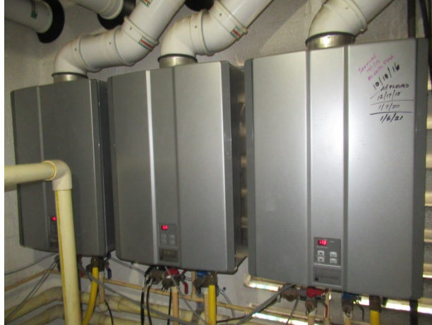
Typical water heaters
