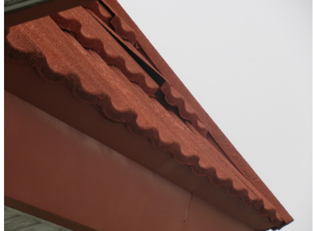
Loose metal sheet
