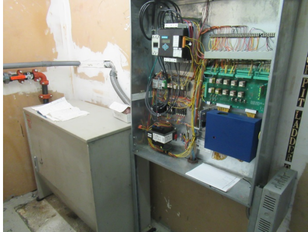
Pump housing and controller
