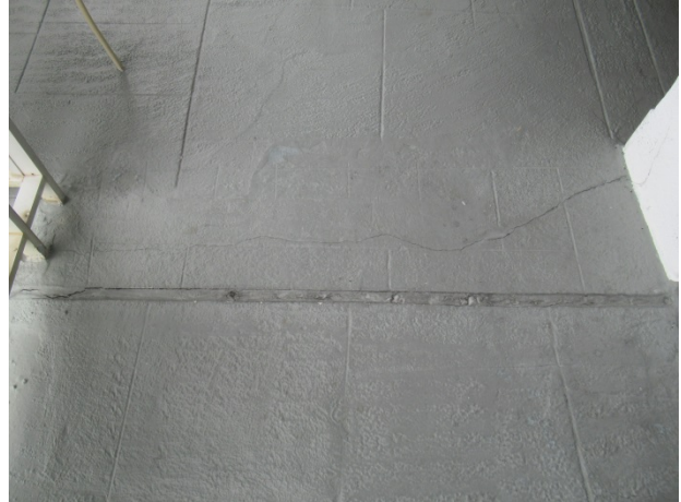
Concrete crack at expansion joint
