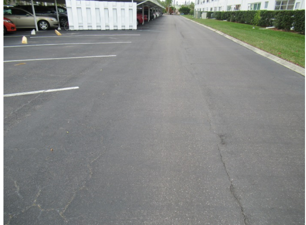
Overview of pavement with cracks
