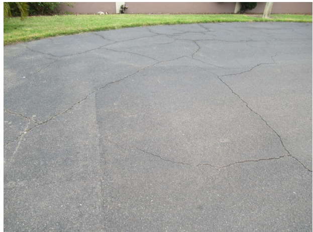
Isolated block cracks
