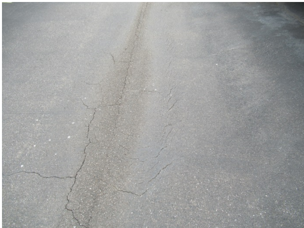
Isolated slippage cracking
