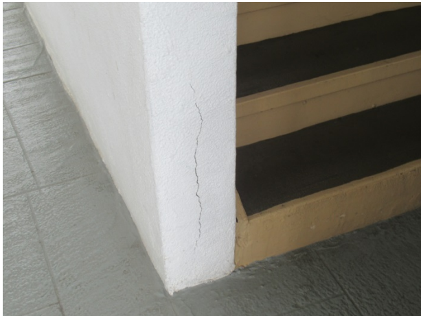
Crack in stucco wall
