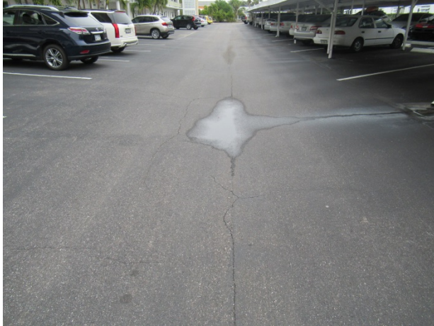
Pavement cracks and standing water
