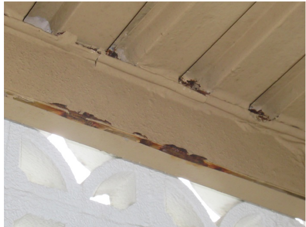
Minor rust at staircase
