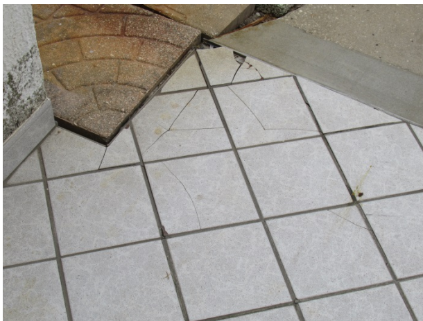
Isolated cracked tiles at first floor
