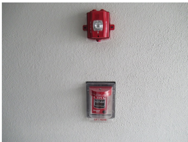
Typical emergency devices
