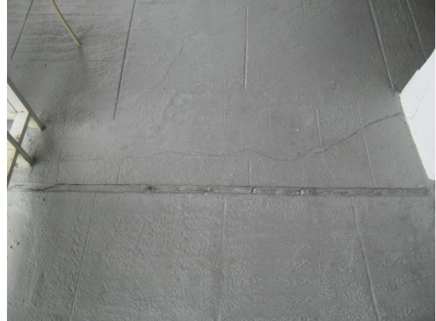
Crack at expansion joint
