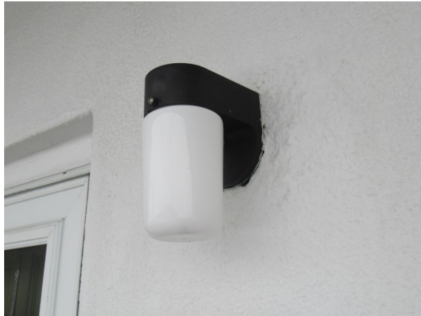
Typical light fixture at unit entrance
