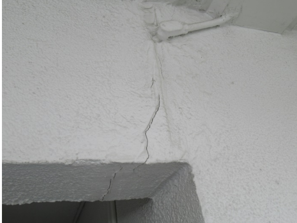
Crack at expansion joint
