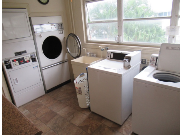
Typical laundry equipment
