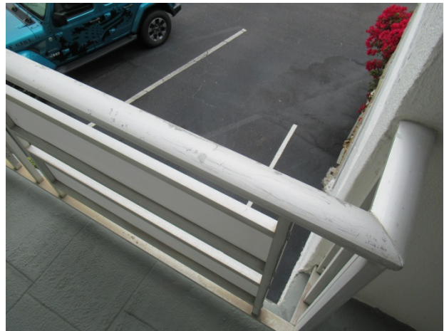
Removed finish and stains
