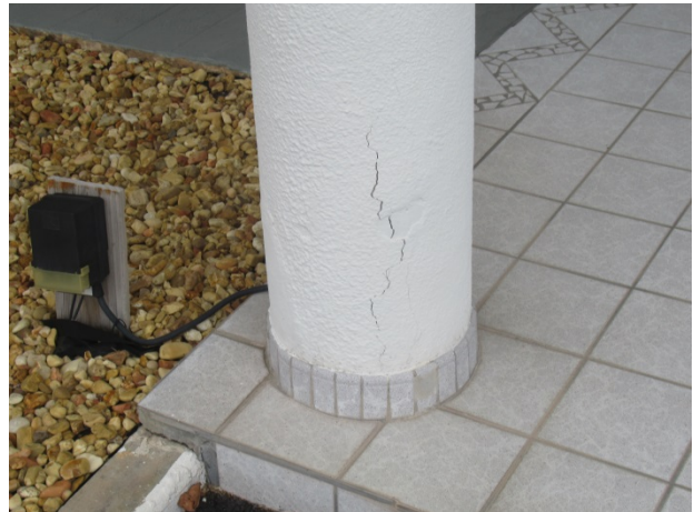
Crack in column
