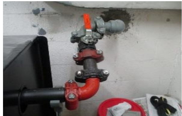
40 Elevator Hydraulic Pump
