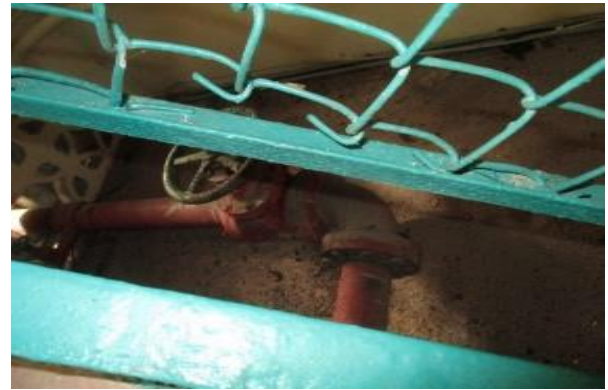
32 Shut Off Valve/s
