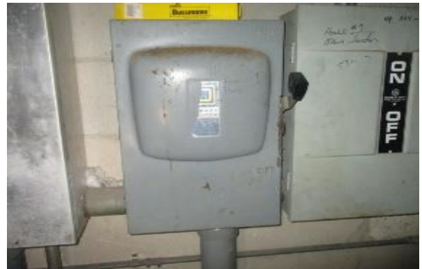
38 Sub Panel Overview
