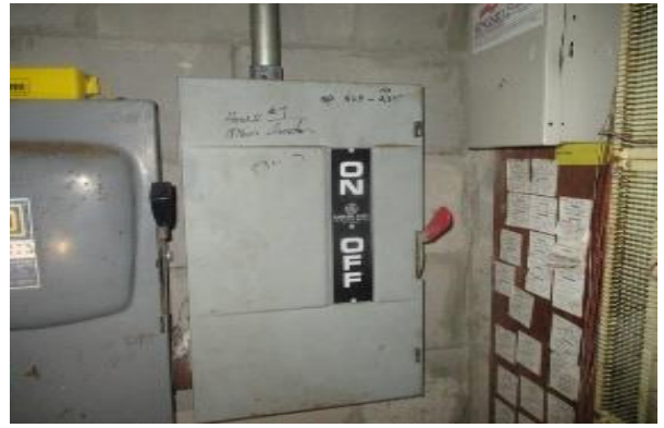
42 Sub Panel Overview
