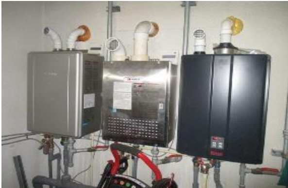
35 Tankless Water Heater/s
