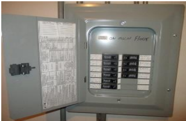
37 Sub Panel Overview
