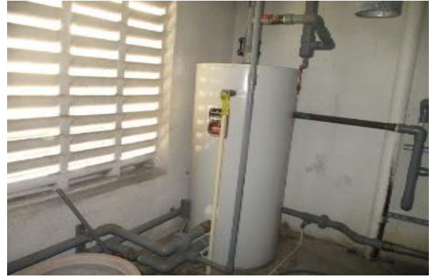
34 Water Heater Overview
