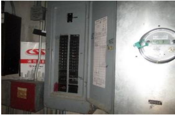
43 Sub Panel Overview
