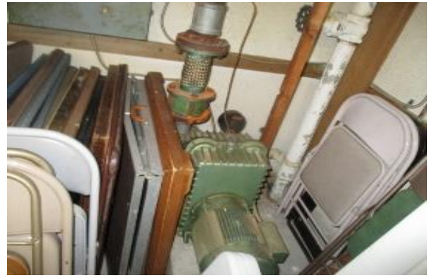
50 Fire Water Pump (Not in Use)
