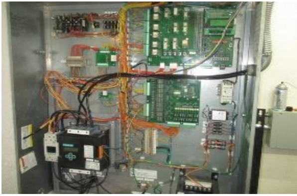
41 Elevator Control Board
