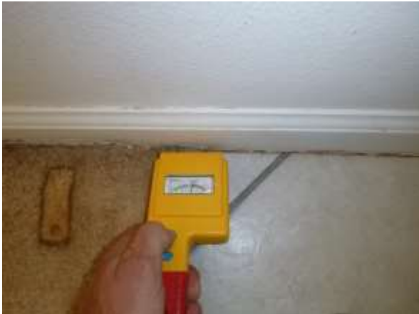
Photo 15: Moisture Reading at Unit 112 Baseboard
