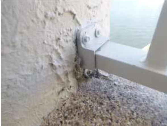
Photo 13: Tear/Void in Walkway Membrane
