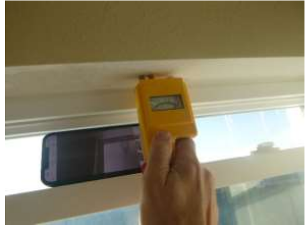
Photo 10: Moisture Reading above Window
