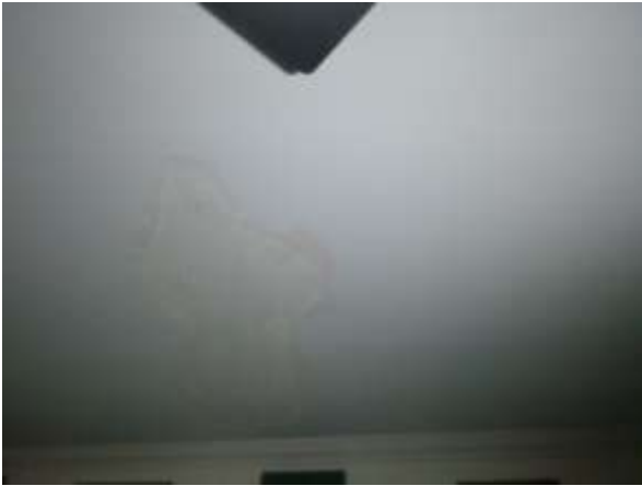
Photo 1: Stain and Crack at Ceiling of Unit 1007
