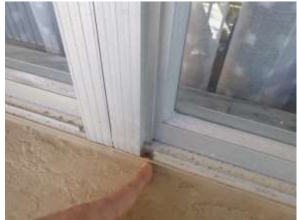
Photo 4: Rusted and Unsealed Window Fastener
