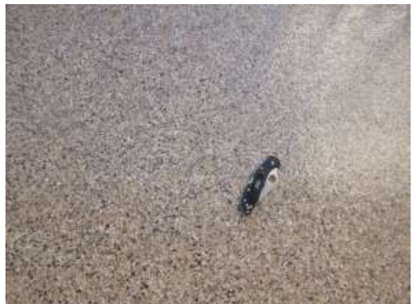
Photo 6: Spall at Walkway Surface
