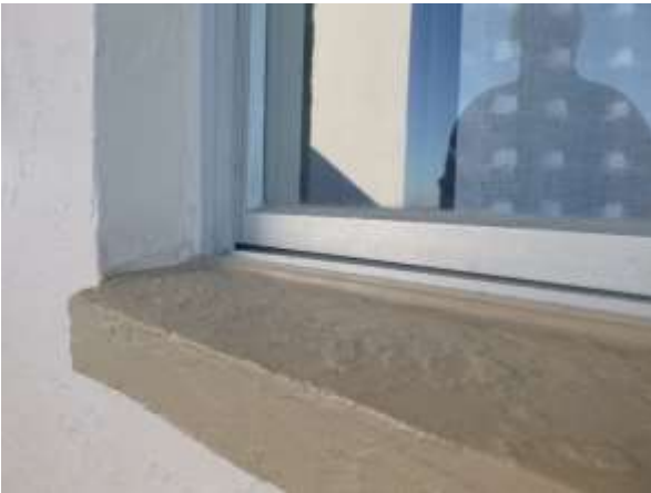
Photo 3: Window not Sealing at PH6
