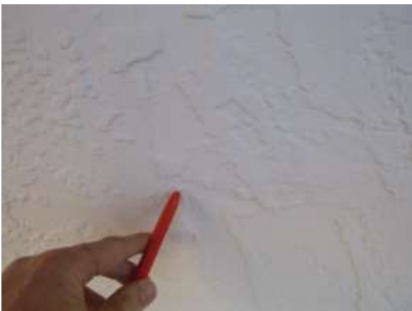
Photo 5: Hairline Stairstep Cracking at Stucco
