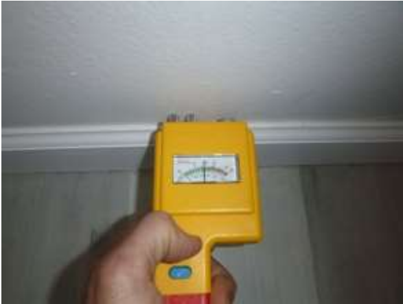
Photo 7: Moisture Reading below Window Mullion
