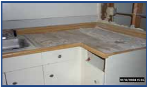
Suspected asbestos-containing materials detected during kitchen renovation project
