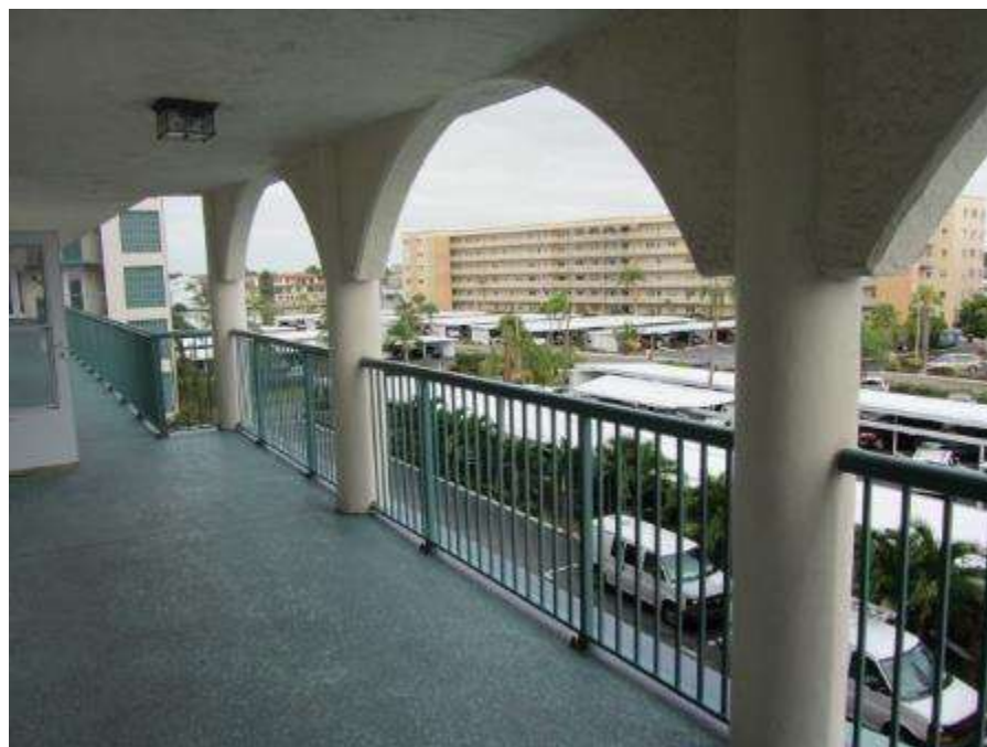
Photo #3 - Overview of common walkway, guardrail, arches, and columns on 4 th floor.
