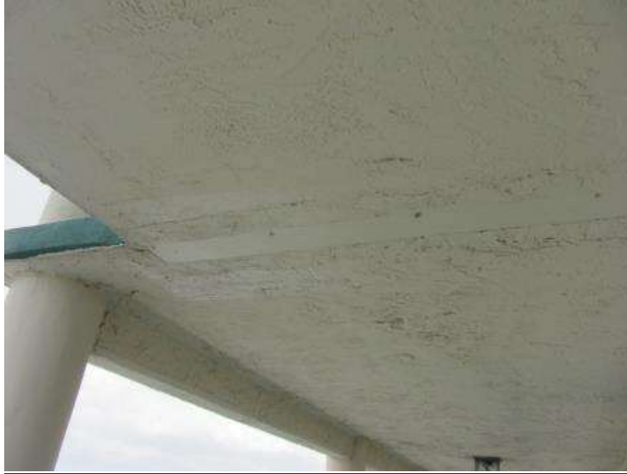
Photo #7 – Underside of typical expansion joint with cover plate attached along one edge
