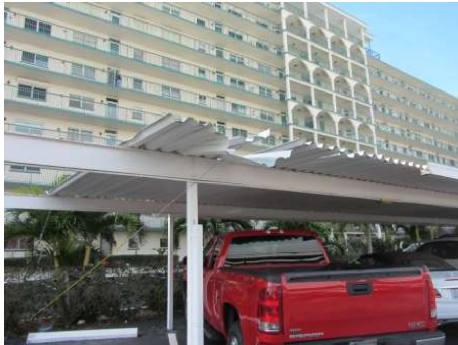
Photo #11 – Damaged carport structure
