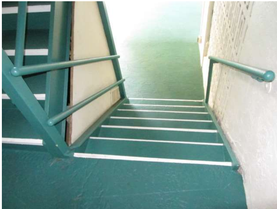
Photo #8 – Typical railings and flight of stairs in partially enclosed stair tower
