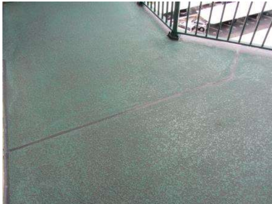
Photo #5 – Top side view of expansion joint at west end of walkway
